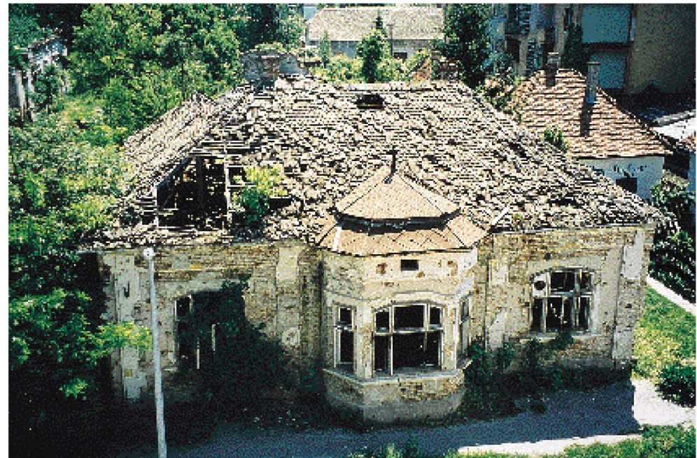
Figure 3: The hospital administration building of Vukovar hospital, which remains in ruins
